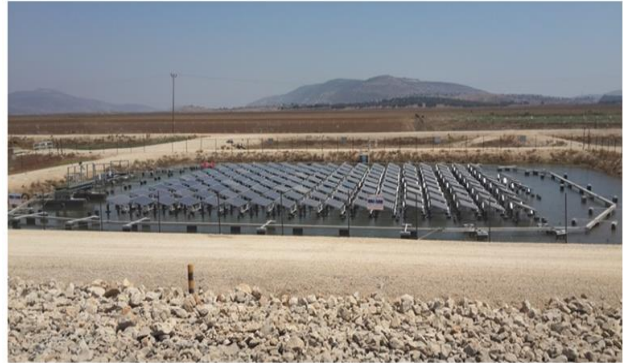
The Solaris Synergy installation on the Eshkol reservoir, Israel
