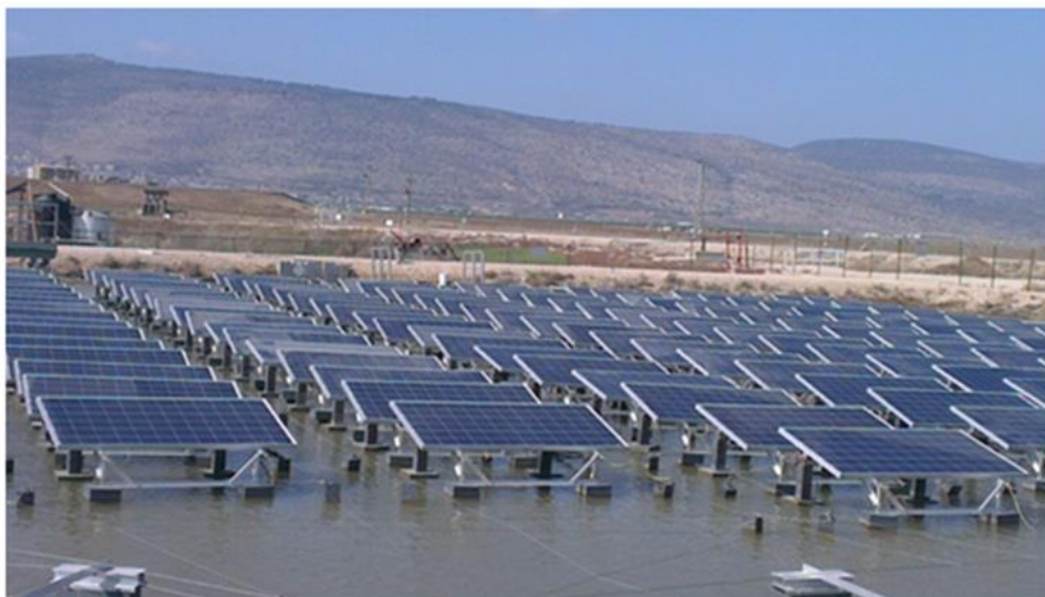
Close-up of the panel floatation system
