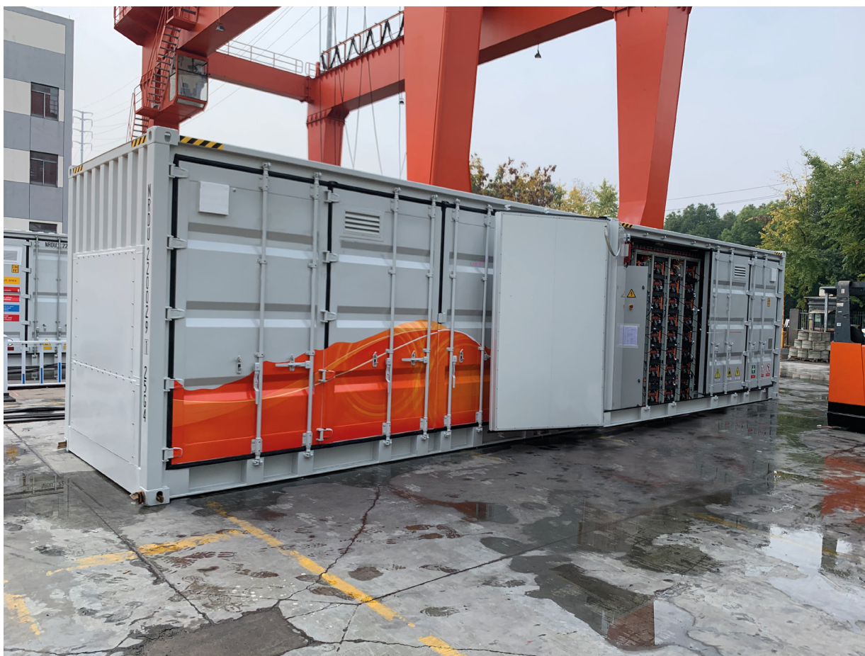
BESS Factory Audit (Source: Sinovoltaics)
