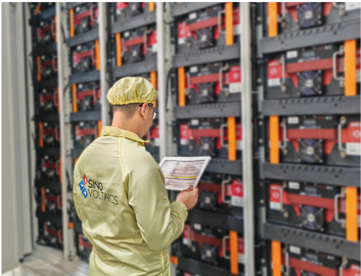
Visual Inspection performed during a FAT (Source: Sinovoltaics 3 )
