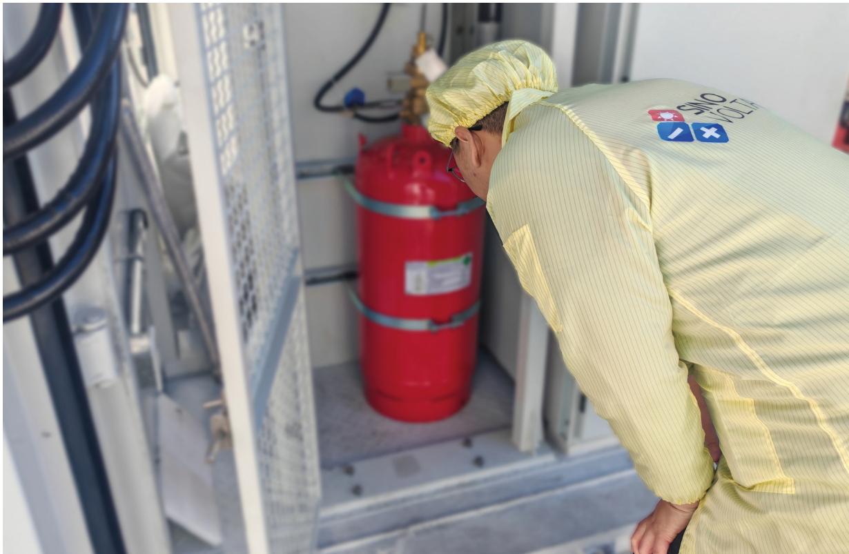
Example of Fire Suppression System Testing Performed During a FAT (Source: Sinovoltaics)
