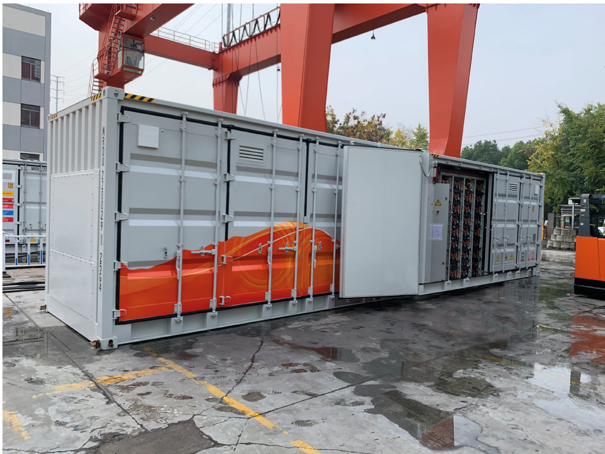
BESS Factory Audit (Source: Sinovoltaics)
