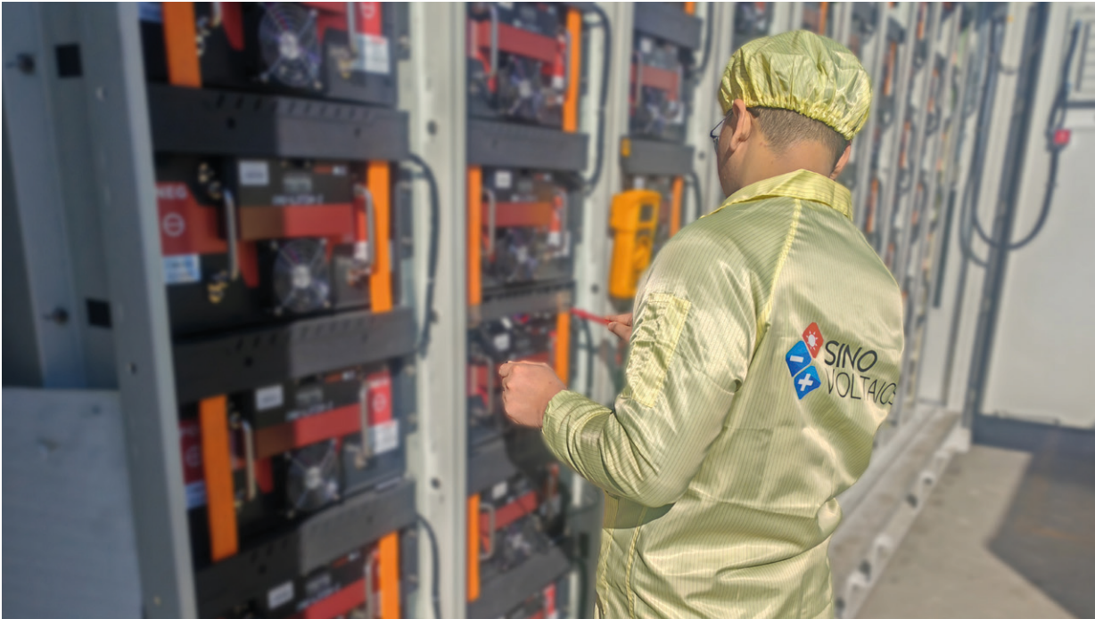
BESS Factory Acceptance Testing (FAT) Electrical Test (Source: Sinovoltaics)
