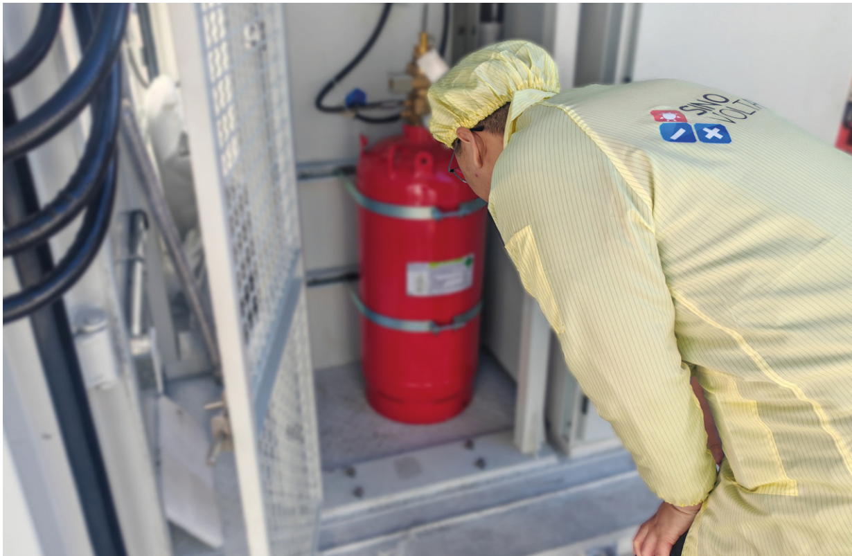
Example of Fire Suppression System Testing Performed During a FAT (Source: Sinovoltaics)
