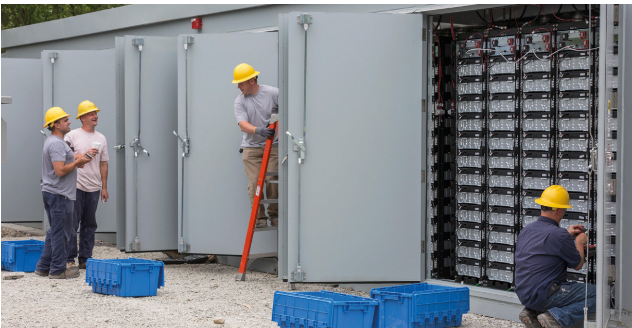
Commissioning team at the site of a battery energy storage system
