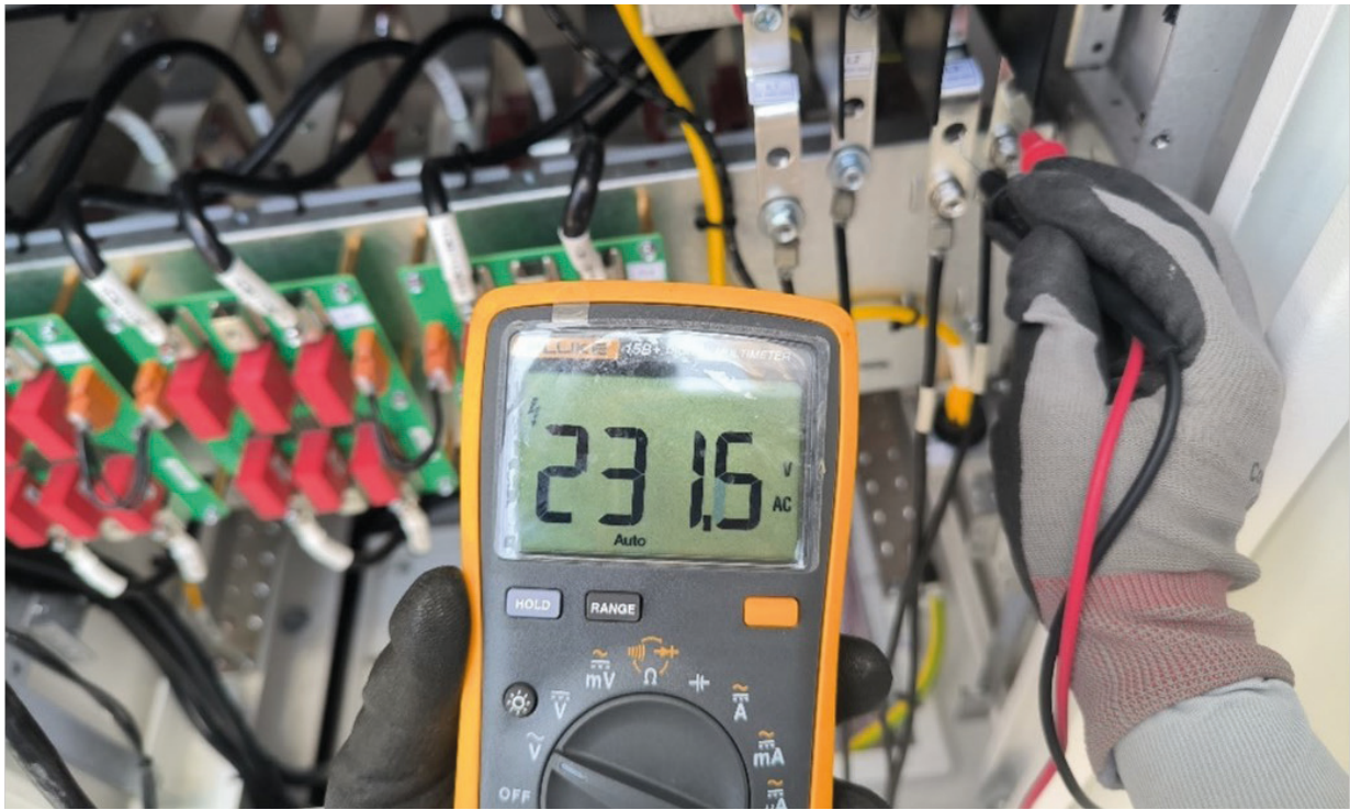
Example of Electrical Measurements done during a FAT (Source: Sinovoltaics 4 )
