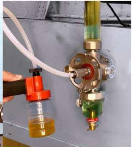
Pulling an Oil Sample
