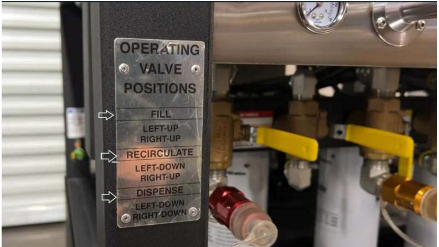
Operating valve positions
