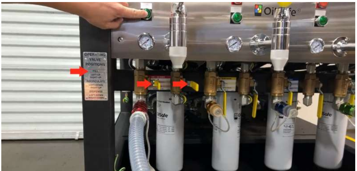
Fill process - both valves in up position
