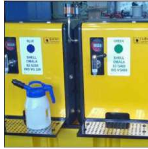
Fig. 9 Lustor Storage System
