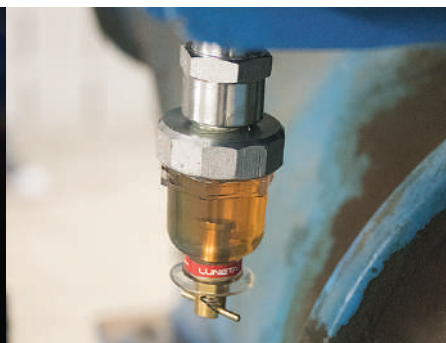
Large Blower - Wastewater Treatment Plant
