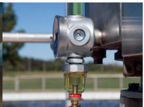
Clarifier - Wastewater Treatment Plant
