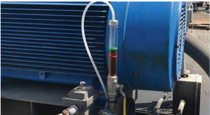
Vent Tube Option - Cooling Tower
