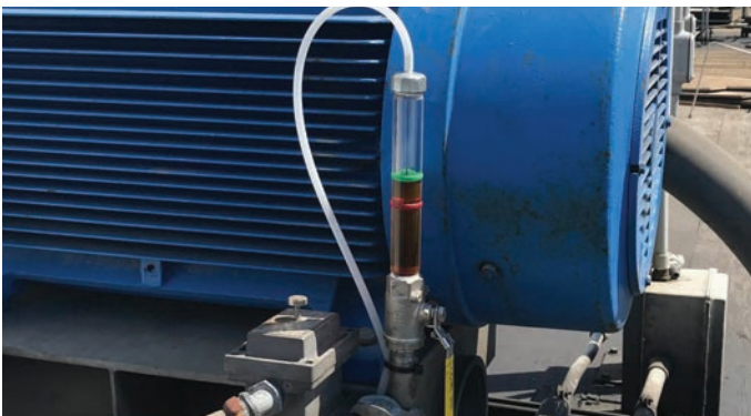
Vent Tube Option - Cooling Tower
