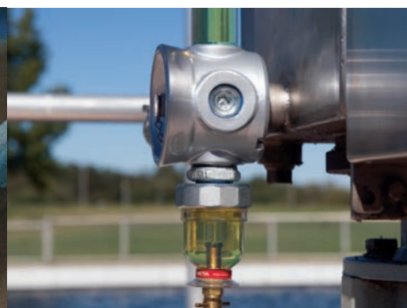
Clarifier - Wastewater Treatment Plant
