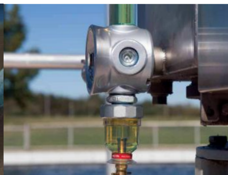
Clarifier - Wastewater Treatment Plant
