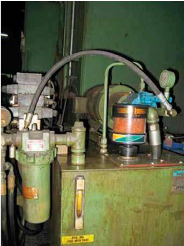
Figure 6. Protection of oil reservoirs with Air Breathers.
