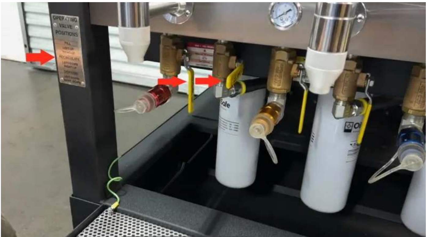
Recirculation process - left valve up and right valve down
