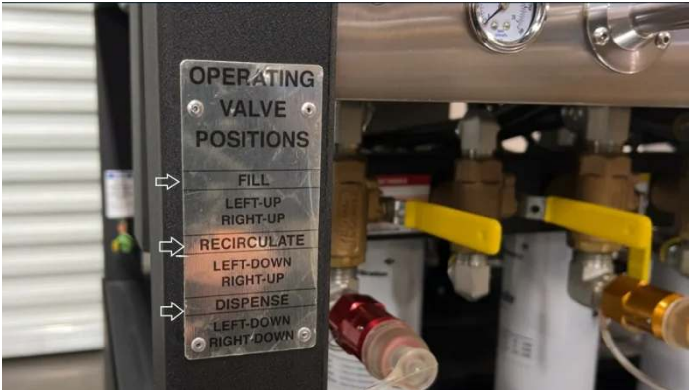
Operating valve positions
