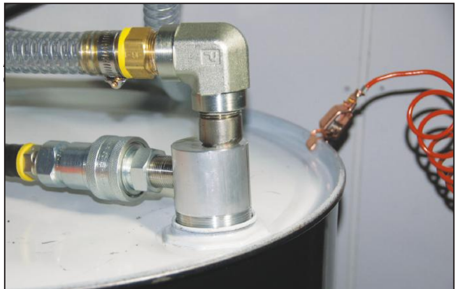
FIGURE 2: Static Discharge Grounding Wire
